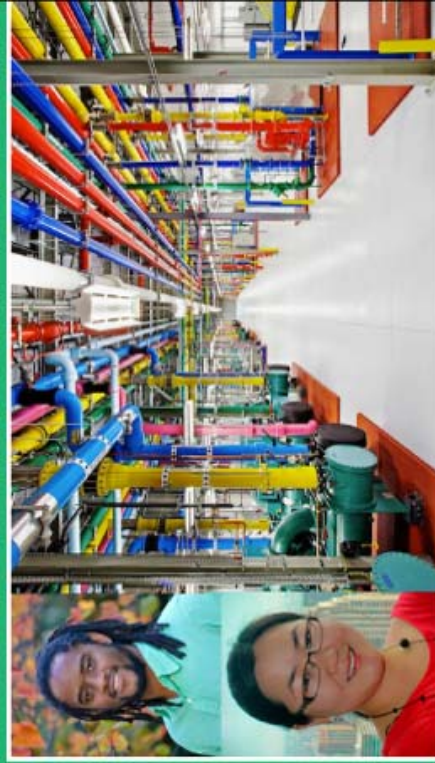
Picture: Jason Mars, Lingjia Tang and Inside Google's Douglas County, Georgia data center
